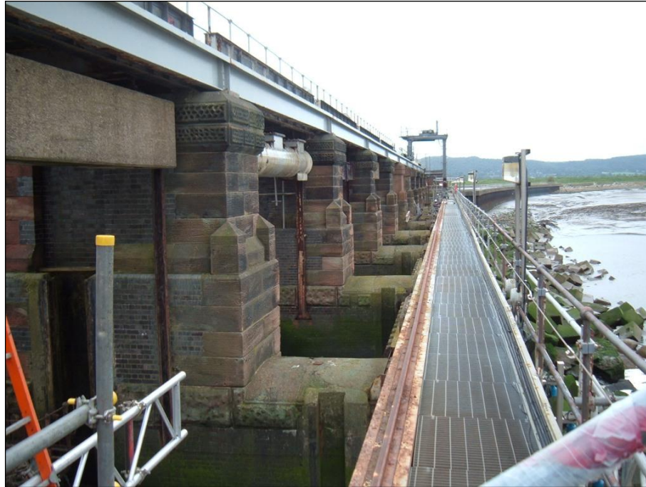
Plate 4. Maintenance works from the low gantry of the Weaver Sluices looking downstream with the river on the right on 12 th September 2010. Completed restoration of the counter weight to one of the sluice gates and replacement of the high gantry framework is shown.
