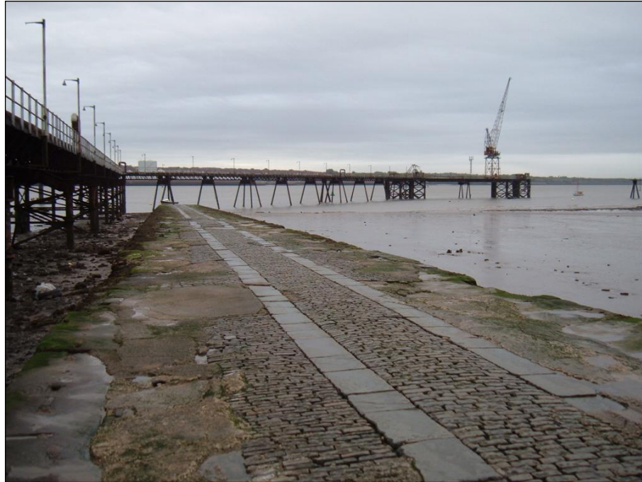
Plate 6. Rock Ferry slipway on 13 th September 2010 showing previous concrete repair work and the derelict tanker cleaning jetty to the left.
