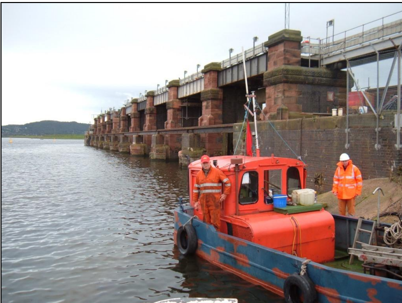
Plate 2. The Weaver sluices viewed from the Manchester Ship Canal looking downstream on 12 th September 2010.
