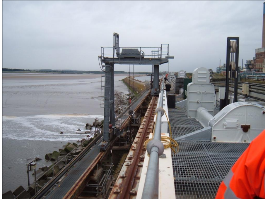
Plate 3. Maintenance works on the high gantry of the Weaver Sluices looking upstream with the river on the left and the Ship Canal on the right of the embankment (centre distance) on 12 th September 2010. Completed restoration of the winding gear to one of the sluice gates and replacement of timber decking with galvanised steel grills is shown.
